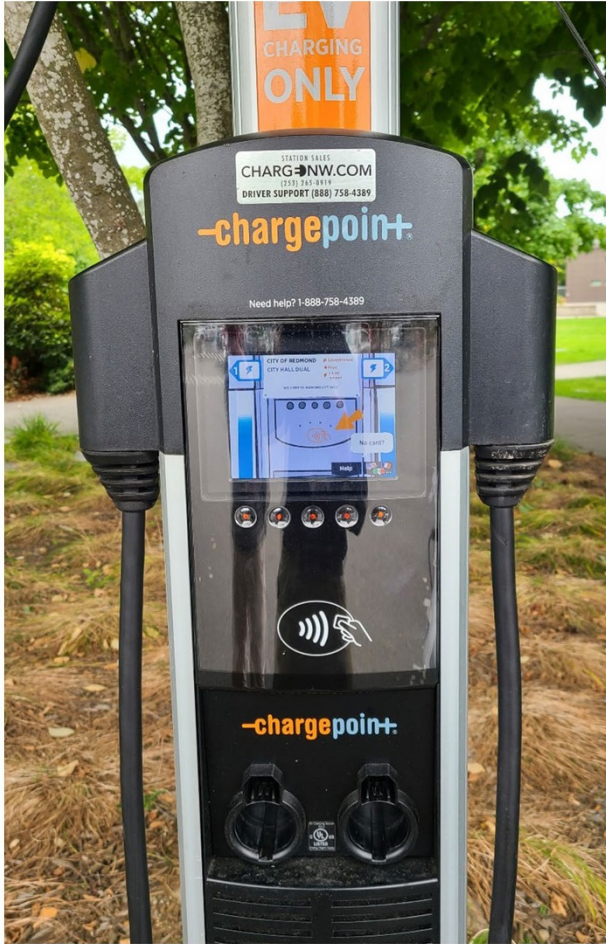
FIGURE 3.3 Free charging station.
