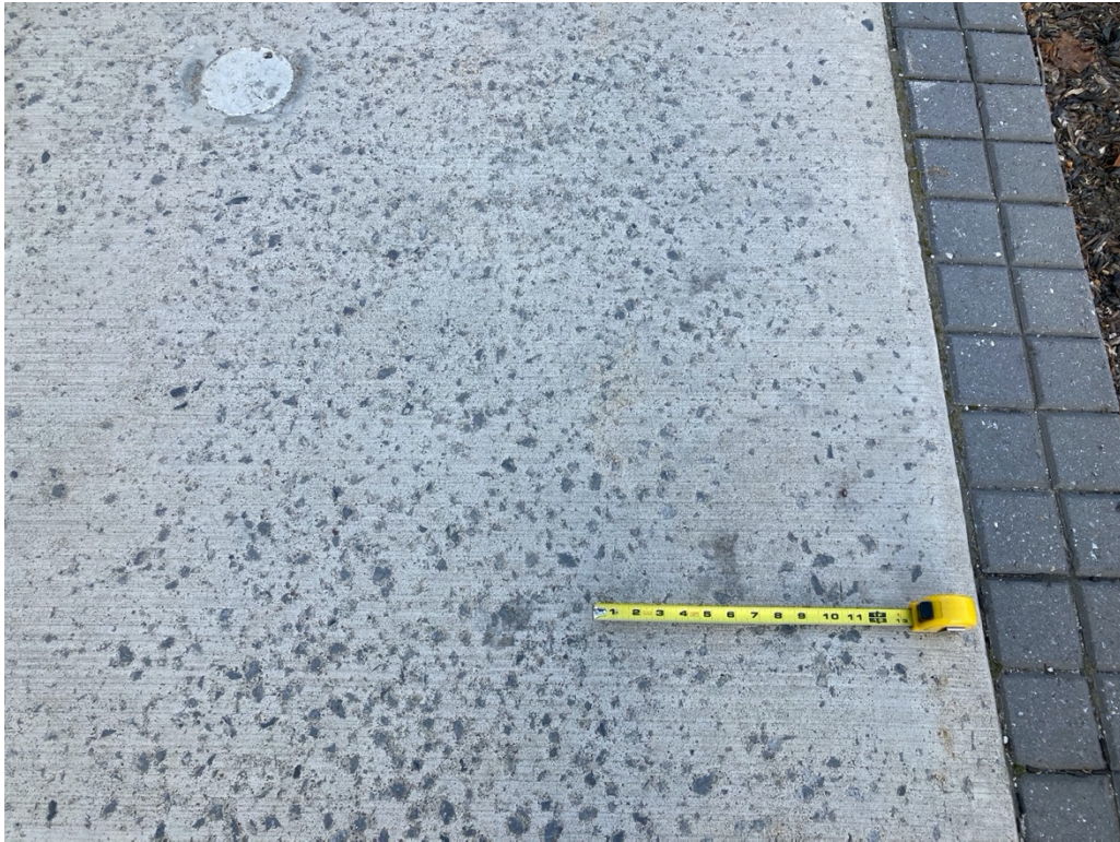
Figure 3. Moderate to severe scaling of the concrete sidewalk
