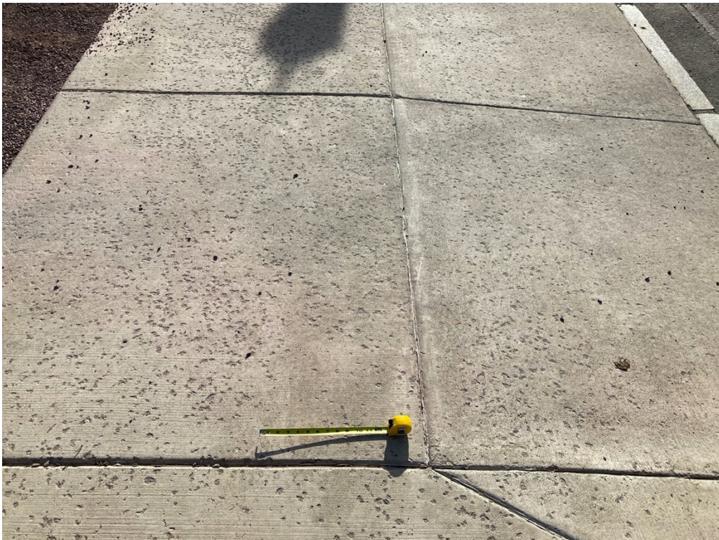
Figure 2. Moderate to severe scaling of the concrete sidewalk. The joint seal has remained in place, preventing penetration of the joints by scaling debris and other incompressible materials.
