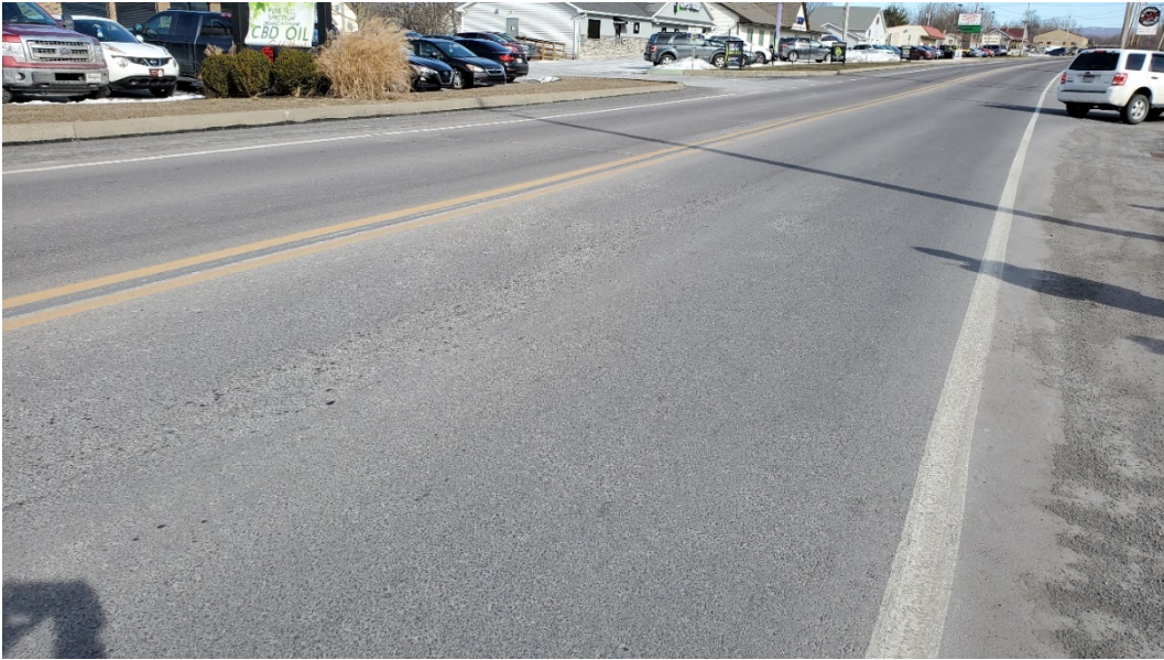
Figure 5. Moderate level of segregated mat on the eastbound lane of SR 1016 – View 1
