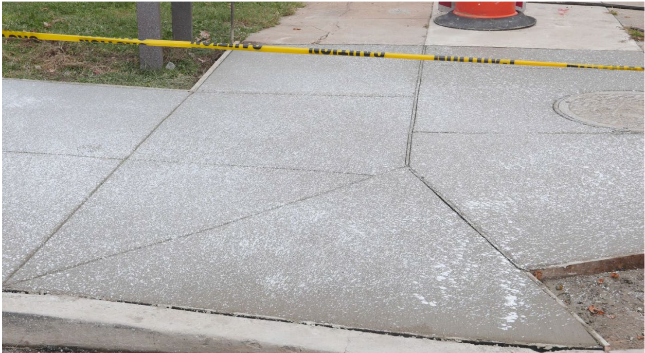
Figure 14. Insufficient application of curing compound results in insufficient curing and ultimately scaling of concrete surfaces (from: [8])
