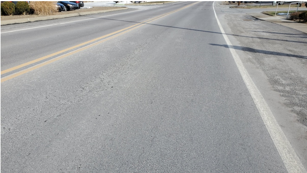
Figure 6. Moderate level of segregated mat on the eastbound lane of SR 1016 – View 1
