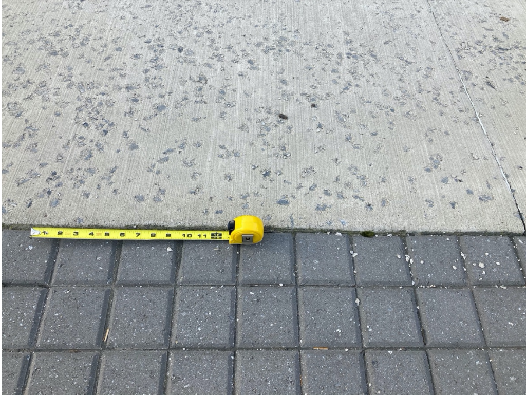
Figure 1. Moderate to severe scaling of the concrete sidewalk. The presence of scaling debris suggests that scaling deteriorations are ongoing.
