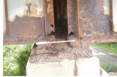
b) Welded patch web plates above bearings at spans 3 and 4 over pier 3 (Bridge D)
