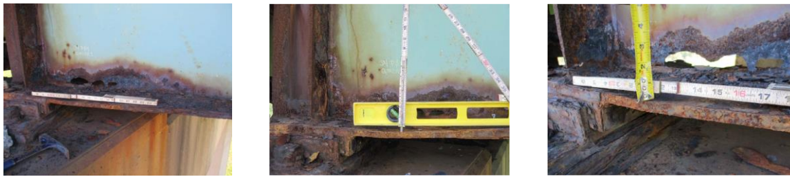
a) Pattern M1 damage (b = 10 in.; a = 2 in.)
