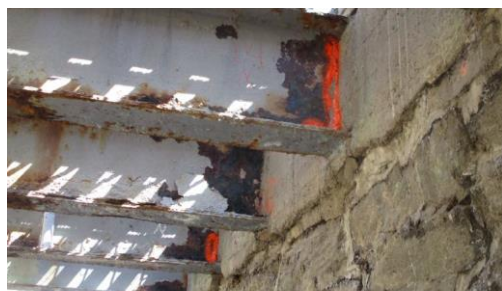
a) beams 4 to 7 reported April 2018
