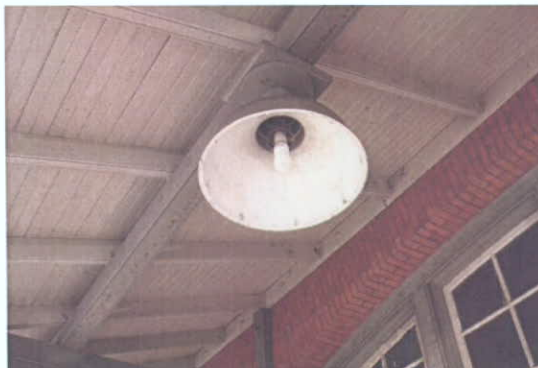
Station building canopy lighting
