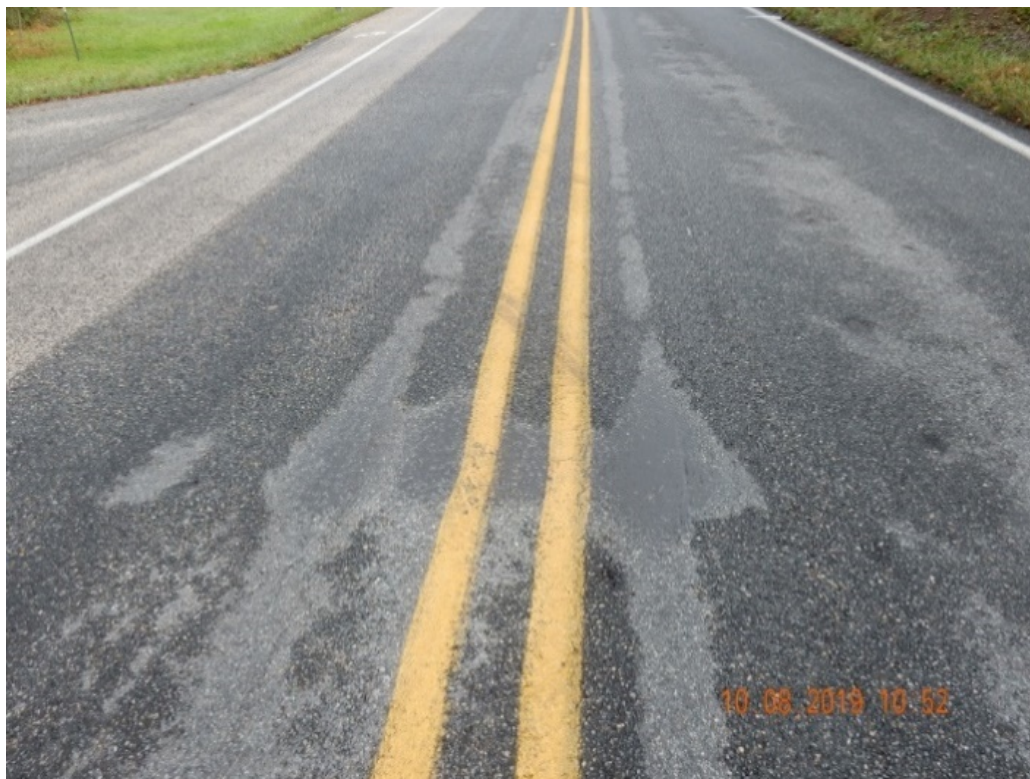
Figure 29. Surface bleeding in the left wheel path.
