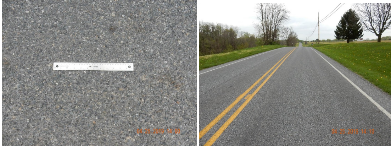
Figure 20. Surface looked good after almost 8 months in service.
