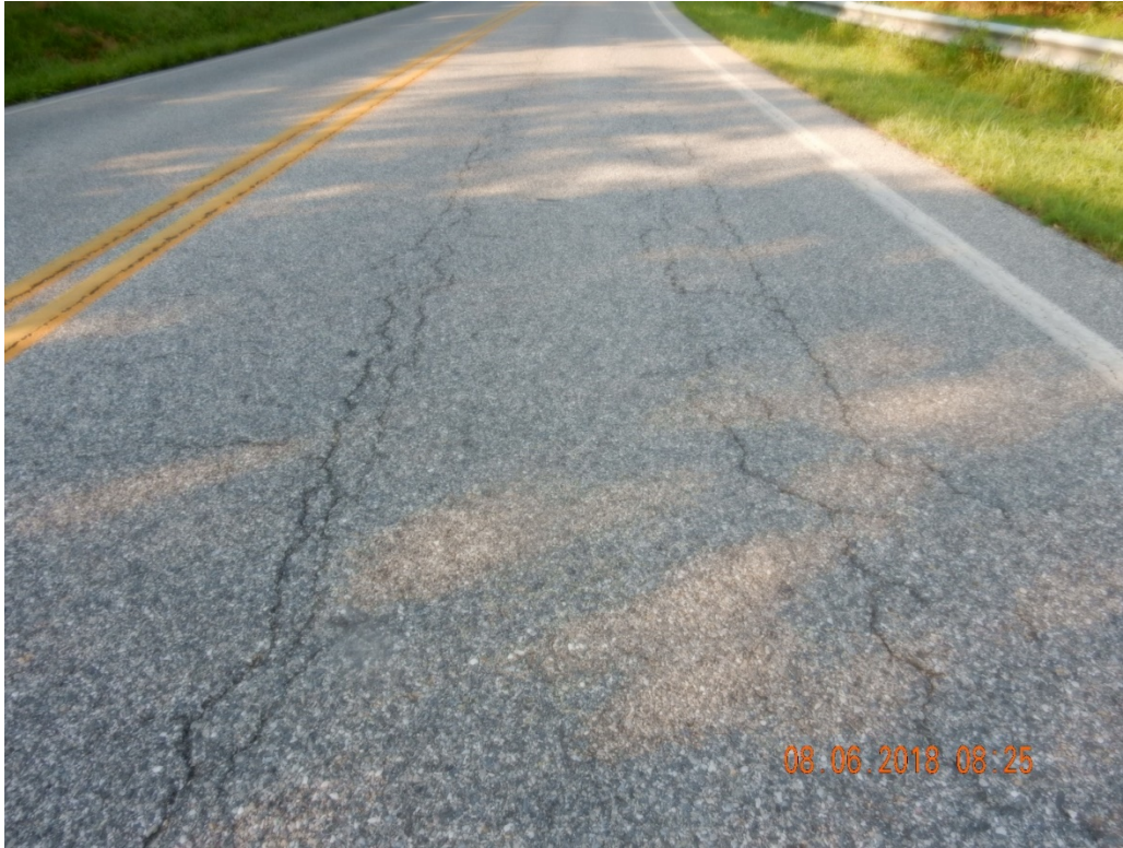
Figure 3. Longitudinal fatigue cracks on the southbound.
