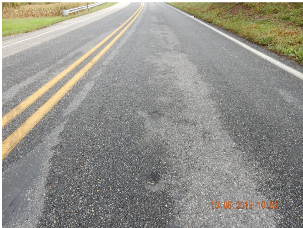
Figure 26. Spots of chip loss to the left of the mat center on the northbound.
