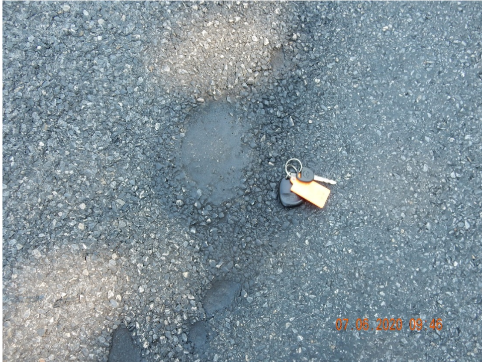
Figure 35. A closeup of the area with material loss and exposure of fabric.
