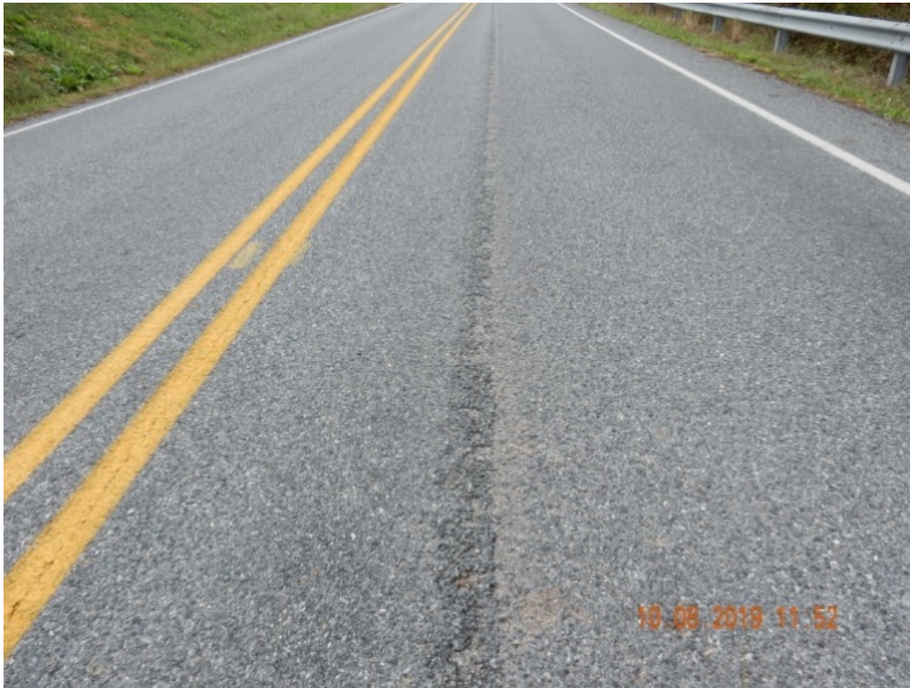
Figure 30. Minor chip loss at the chip seal joint.
