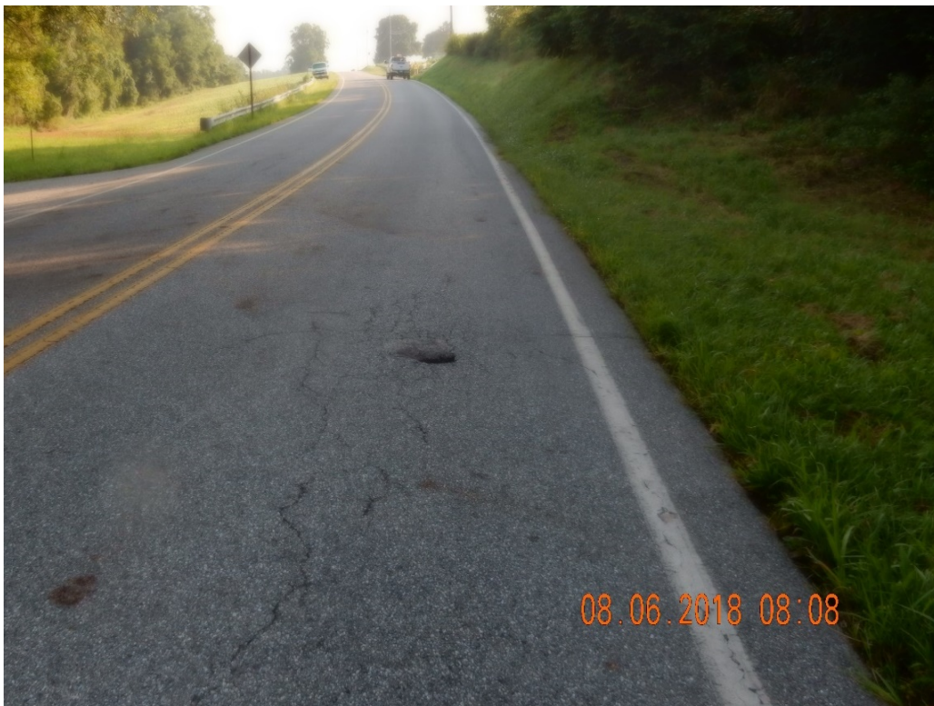
Figure 2. Alligator fatigue cracks on the northbound.
