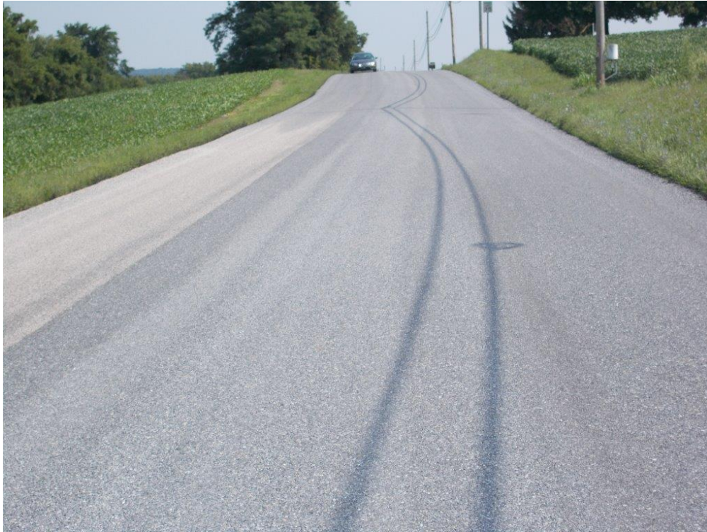
Figure 15. General appearance of the mat after eight days in service looking northbound.
