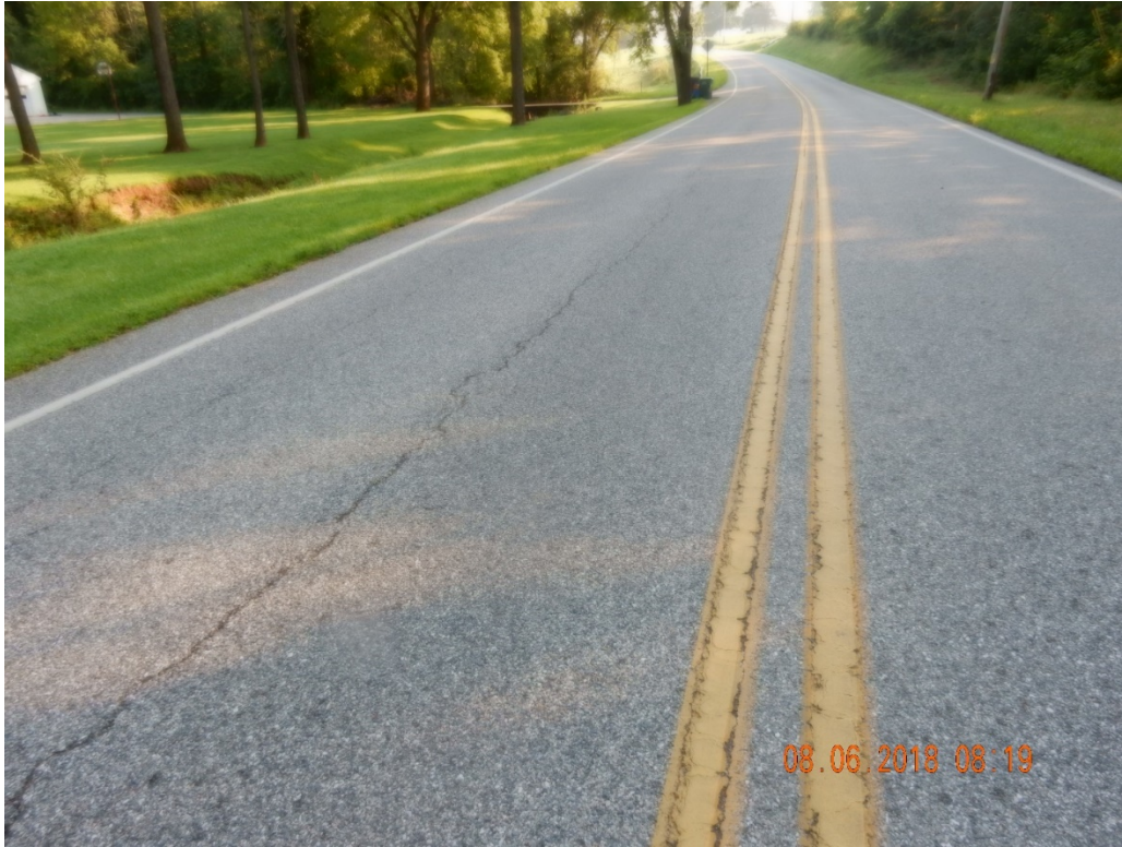
Figure 1. Longitudinal crack at the center of the mat on the southbound.
