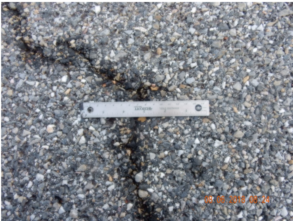
Figure 4. Cracks were mostly 1/8- to 1/4-inch wide.
