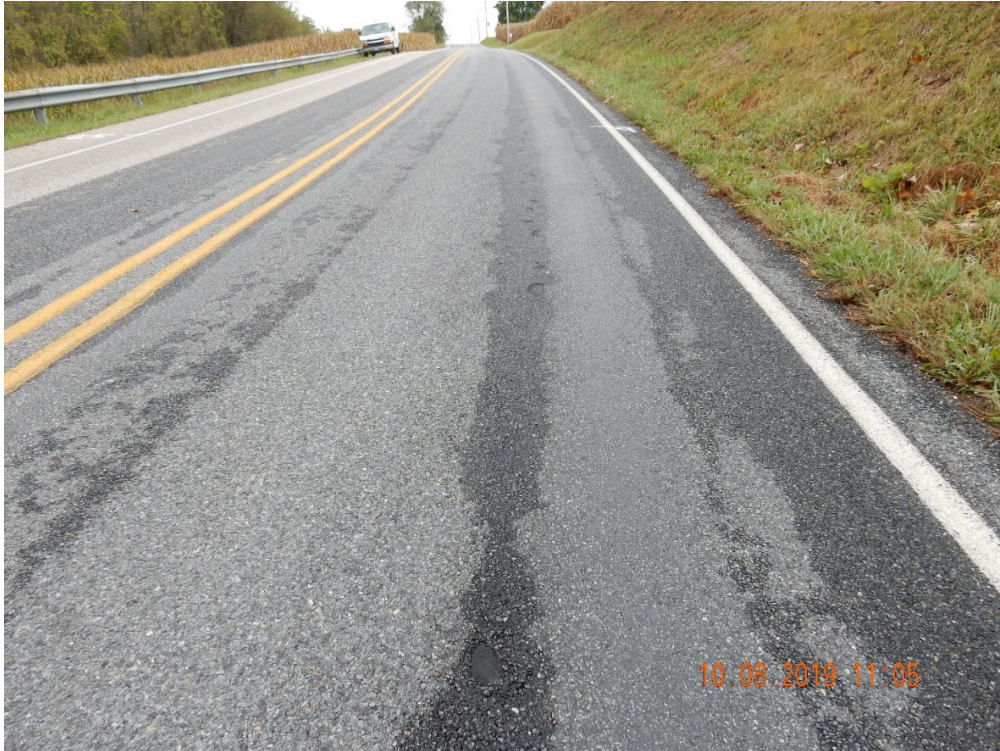
Figure 25. Spots of chip loss to the right of the mat center on the northbound.
