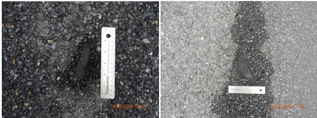
Figure 22. Spots of chip loss and the bubbled up exposed geofabric.
