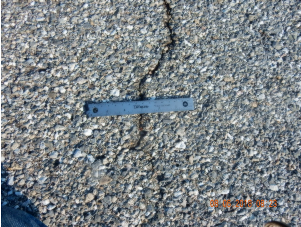
Figure 5. Another closeup view of surface cracks.
