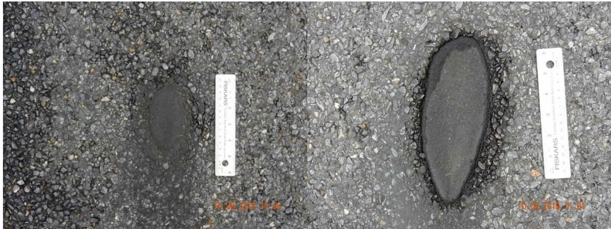
Figure 23. Additional spots of chip loss and the bubbled up exposed geofabric.
