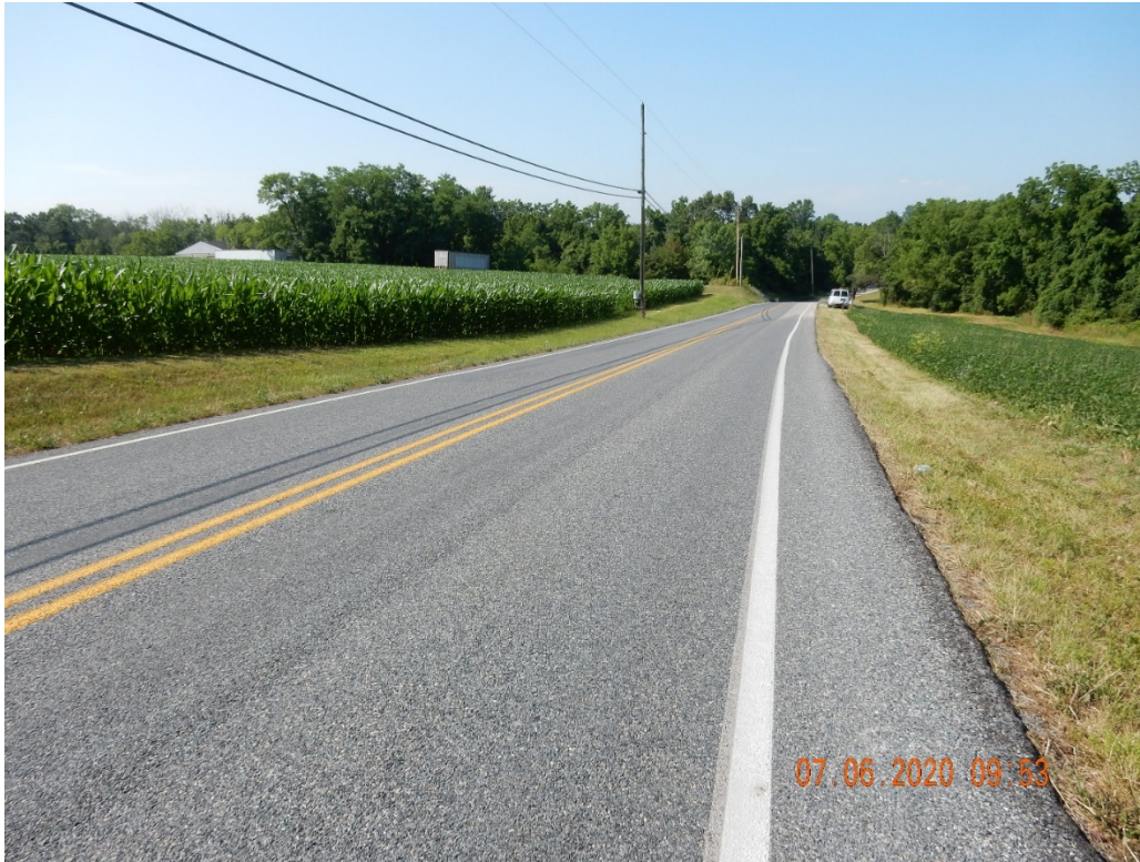
Figure 32. The surface generally looked good after two years (looking southbound).
