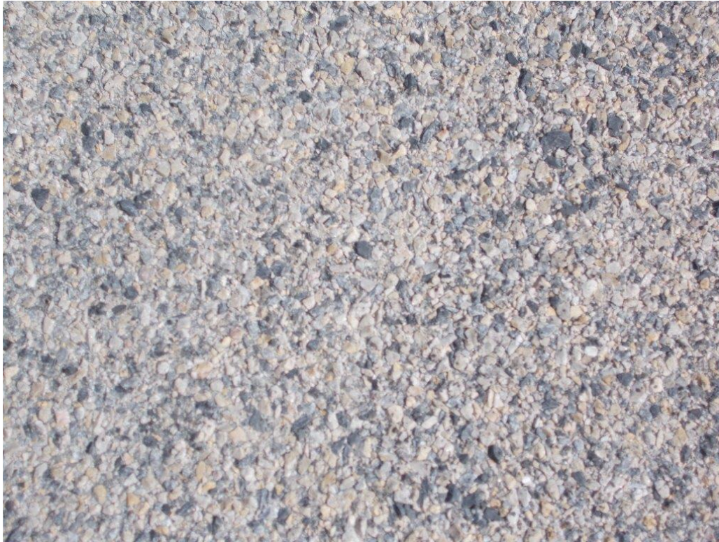
Figure 16. Tight texture of the mat after 8 days in service.
