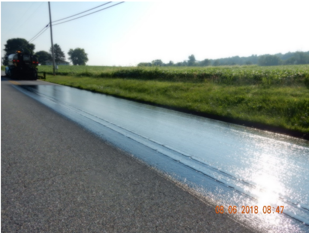
Figure 7. PG 70-22 asphalt placed on a section of the road on the northbound.
