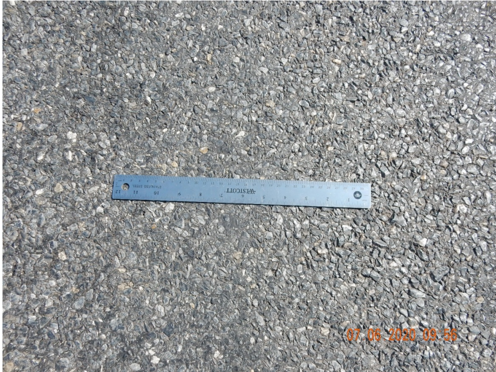
Figure 33. Except several distressed areas, the mat texture looked in very good shape.
