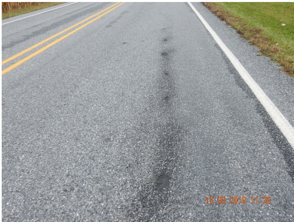
Figure 24. Spots of chip loss to the right of the mat center.
