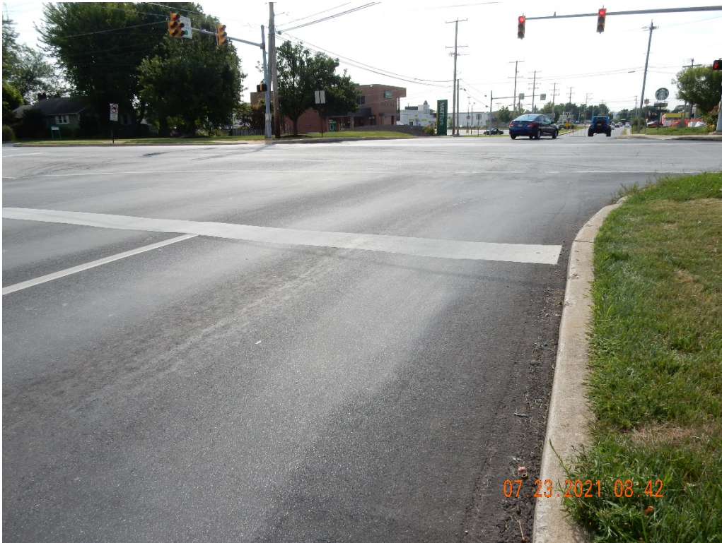
Figure 23. Minor rutting and bleeding on the southbound lane at the intersection.
