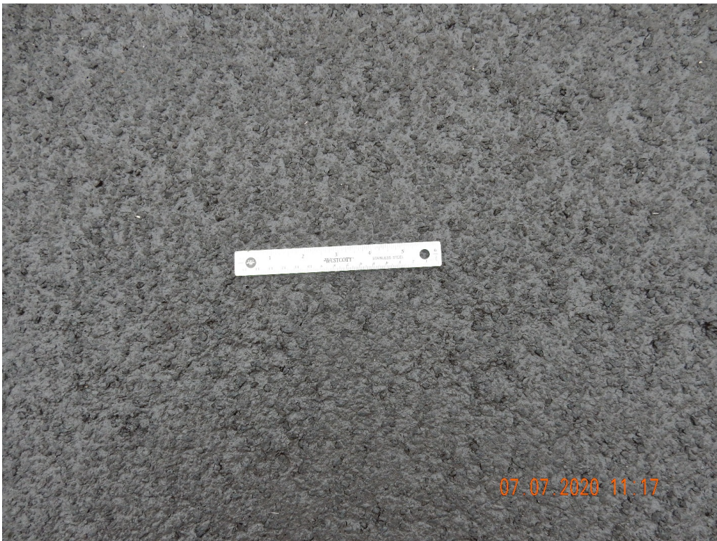
Figure 9. A close-up view of the micro surfacing texture on the northbound lane.
