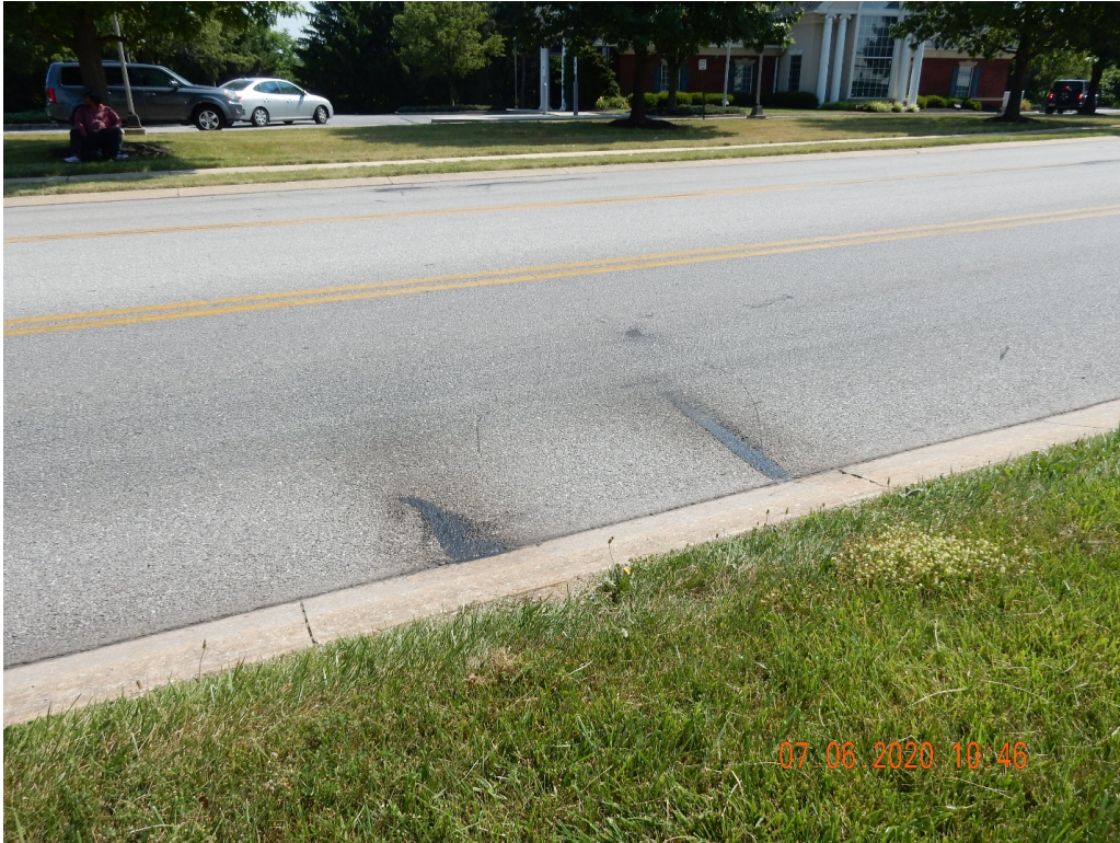
Figure 3. Southbound with sealed transverse cracks.
