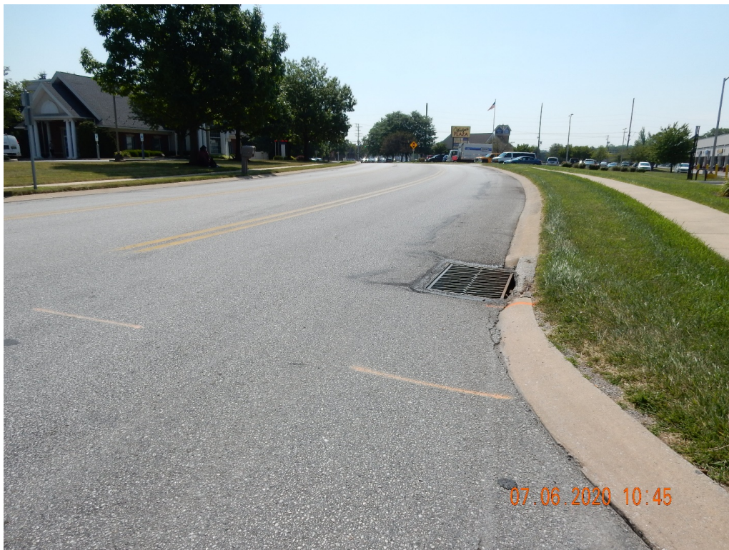
Figure 2. General view of the existing pavement (picture taken at intersection with Trolley Road).
