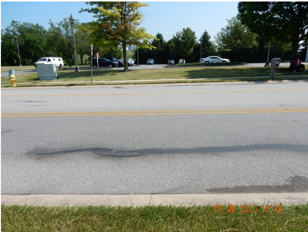
Figure 4. Southbound with sealed longitudinal cracks.
