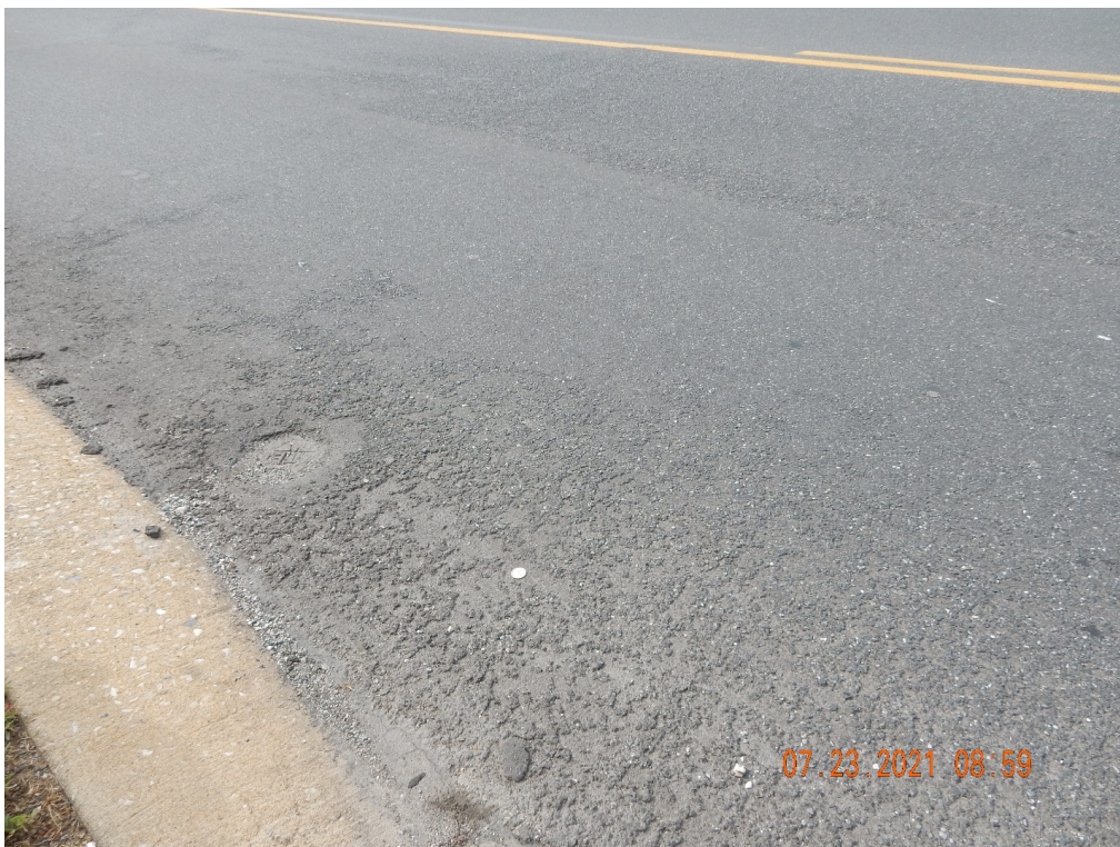
Figure 24. Localized loss of material on the northbound lane at the intersection with Trolley Road, possibly because of inadequate application or compaction.
