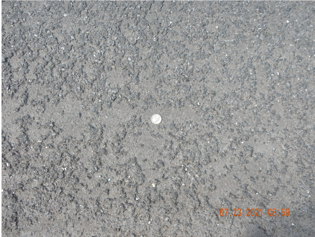
Figure 25. A close-up view of the localized material loss on the northbound lane at intersection with Trolley Road.
