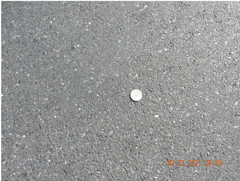
Figure 16. A close-up view of the surface texture on the southbound one year after placement.
