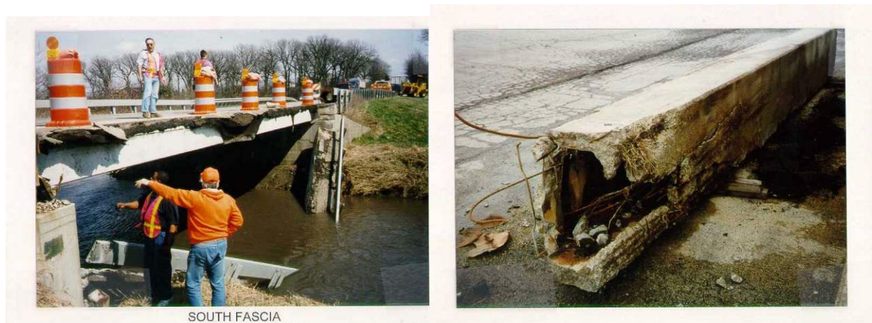
Figure 5: IDOT Structure 046-0055 Beam Failure [046-0055.ppt]
