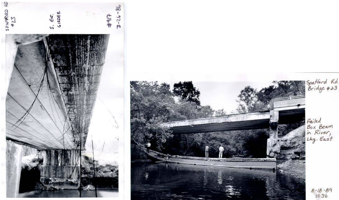
Figure 1: Cuyahoga County Bridge Failure
