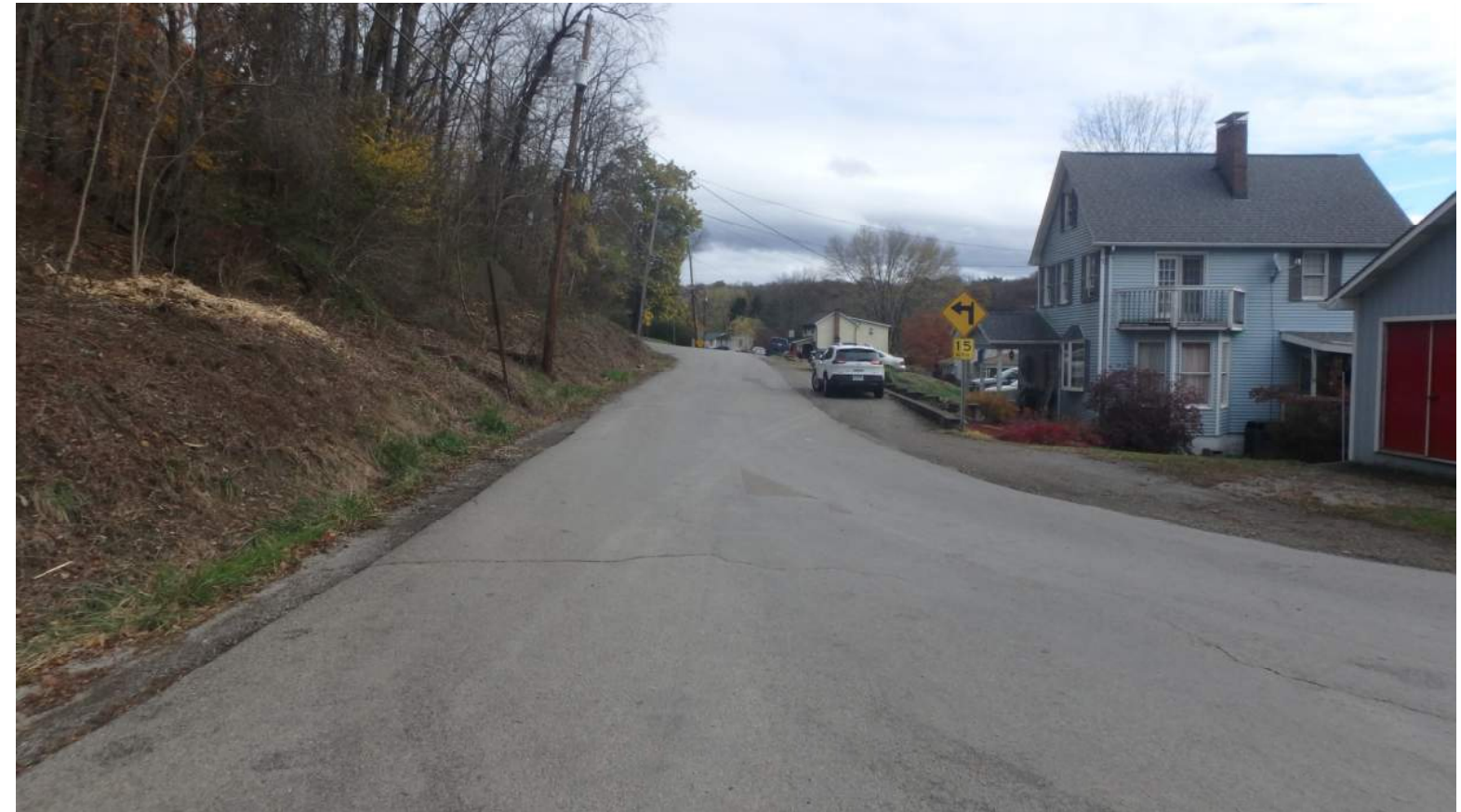
Looking East on SR 2047 (Edmon Rd) Armstrong Co (Cut Left Hill, Widen Road, Improve Drainage)
