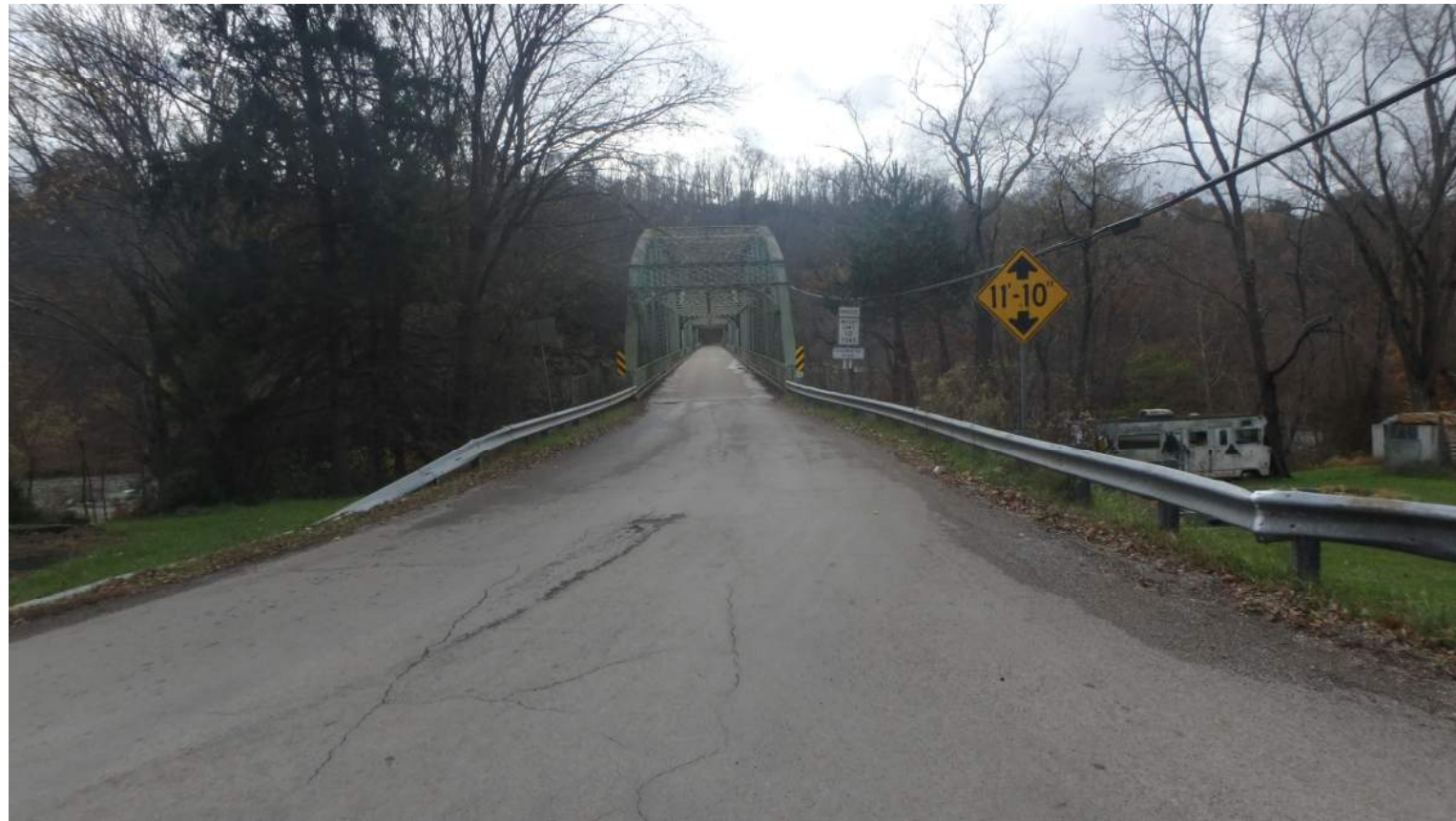
Looking South on SR 1060 (Bridge St) towards Westmoreland Co (Existing T Intersection, Narrow, Posted Bridge)
