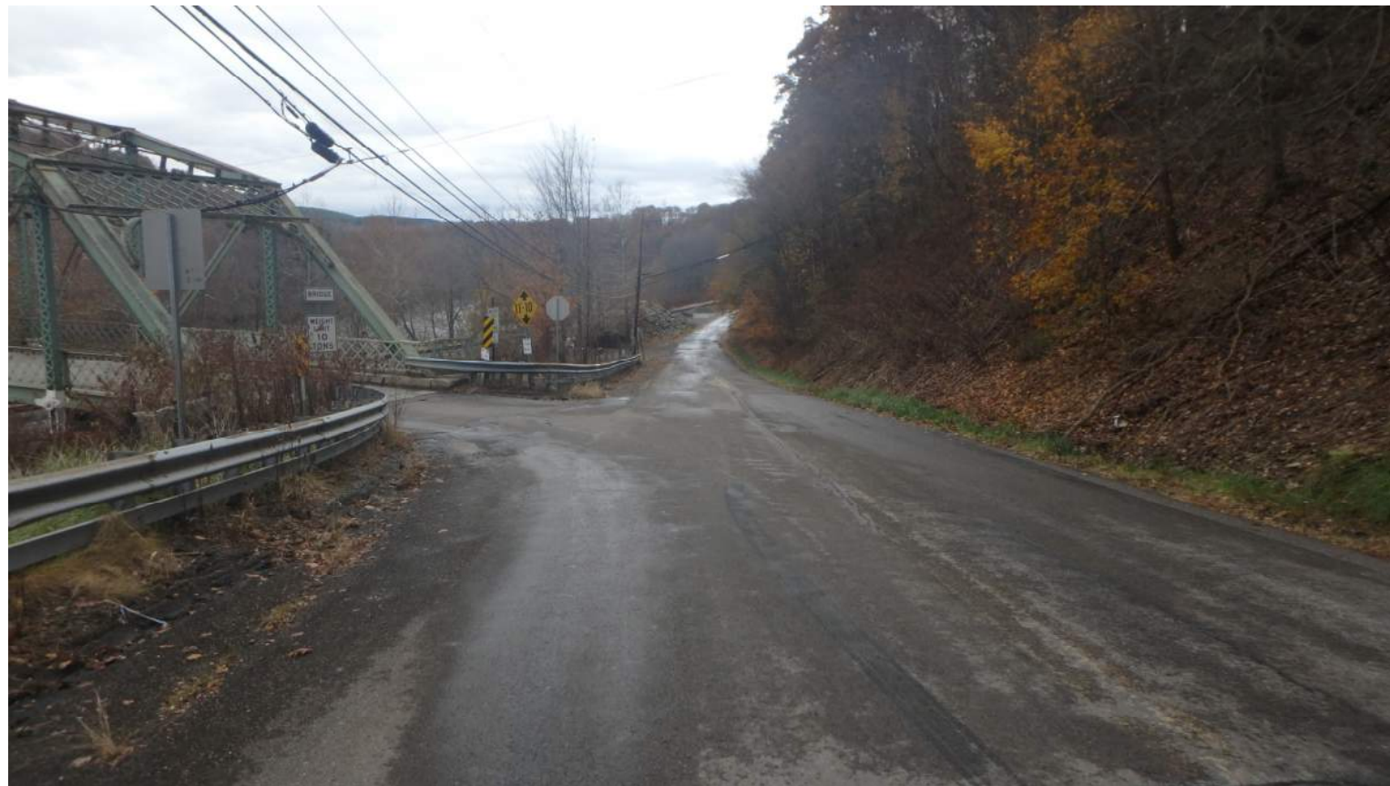
Looking East on SR 1060 (Main St) Westmoreland Co (Full Depth Reconstruction Using Temp Signal/Partial Width, Barrier Wall on Left, Improve Drainage, Relocate Utilities)
