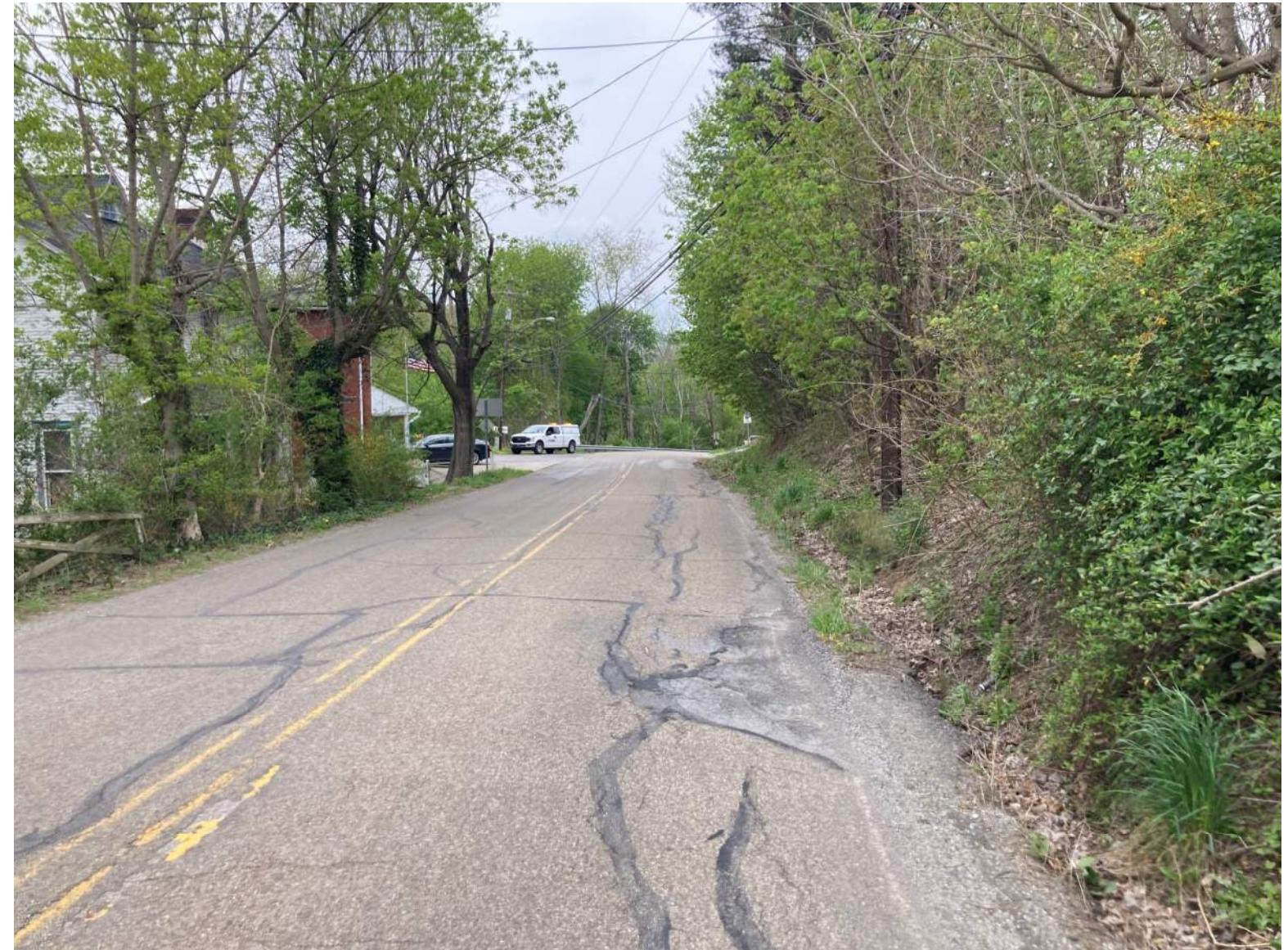
Looking East on SR 1060 (Main St) Westmoreland Co (Full Depth Reconstruction, Short Term Operations, Improve Drainage)
