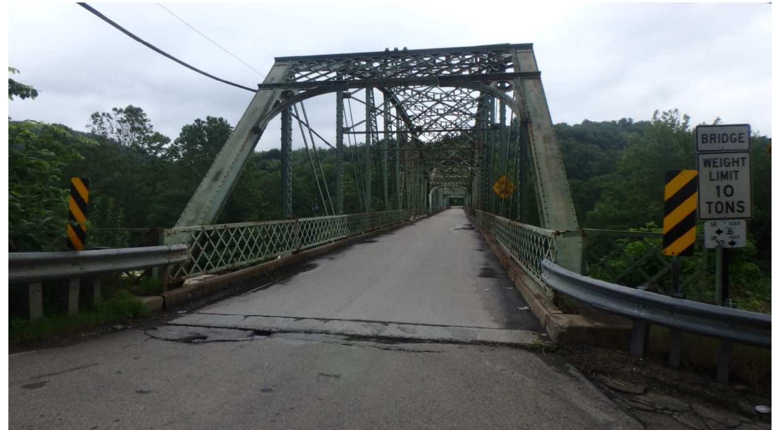
Looking North on SR 1060 (Bridge St) towards Armstrong Co (Existing T Intersection, Narrow, Posted Bridge)
