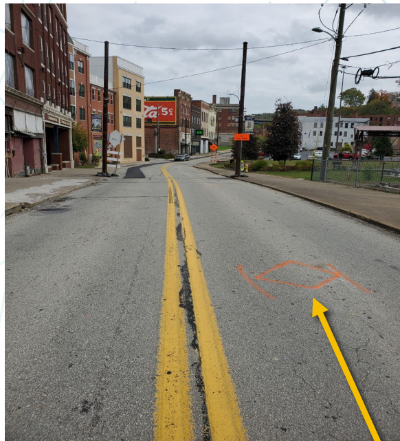
Verizon fiber lines (in pavement)
