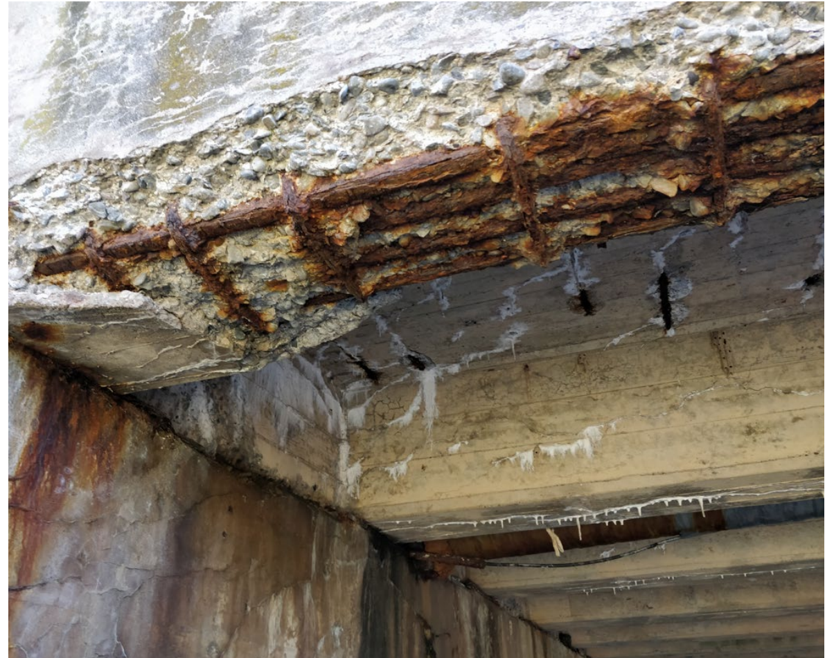
Beaver Run Abutment & Beam Cracks
