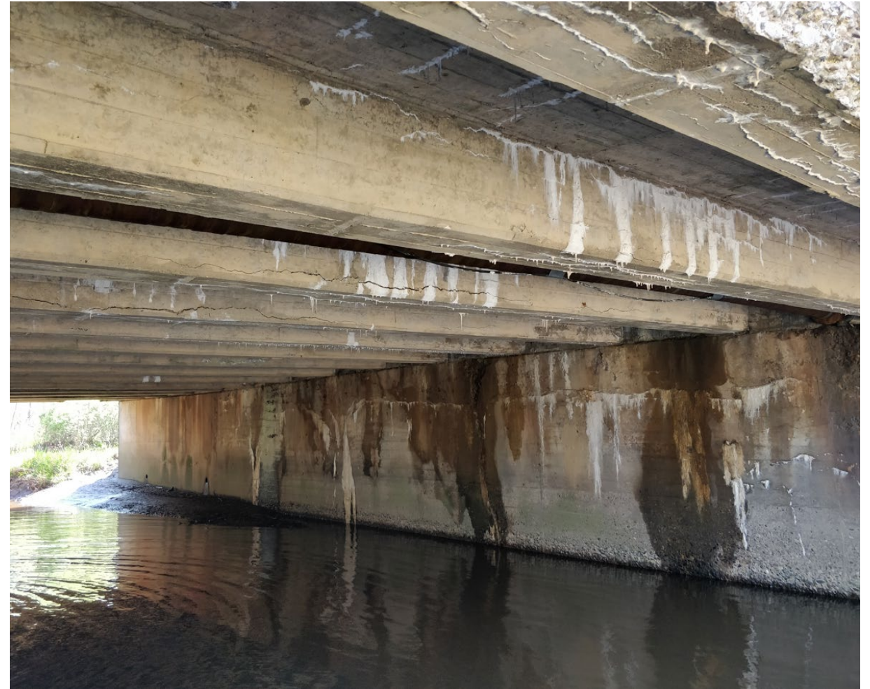
Morgan Creek Abutment & Beam Cracks
