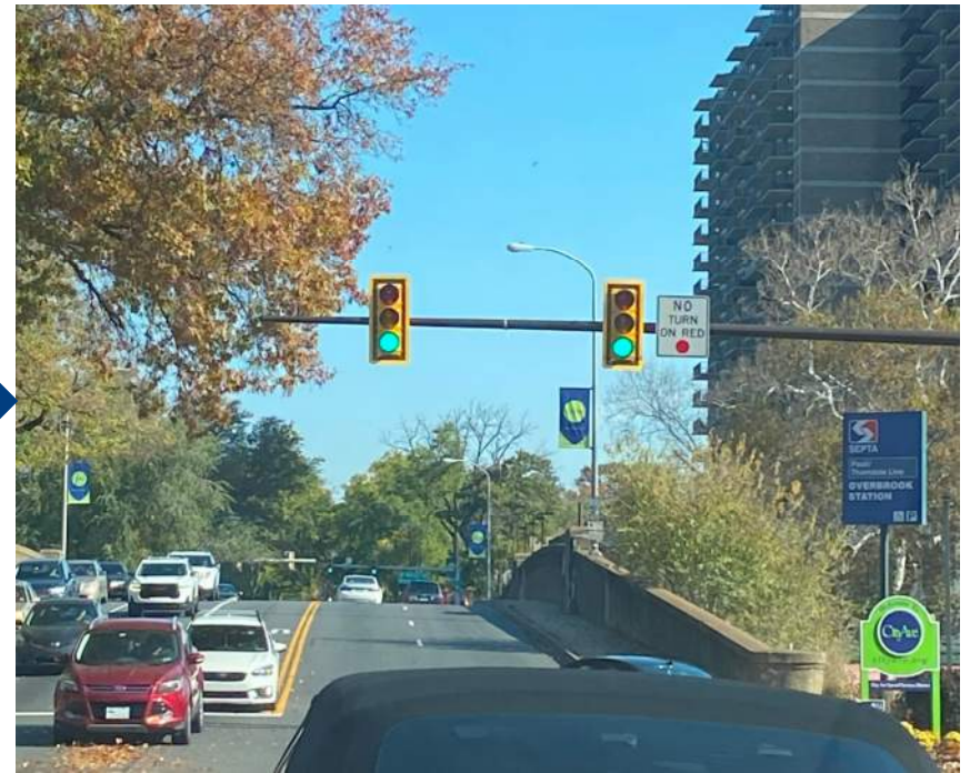
Mast Arm Signals
